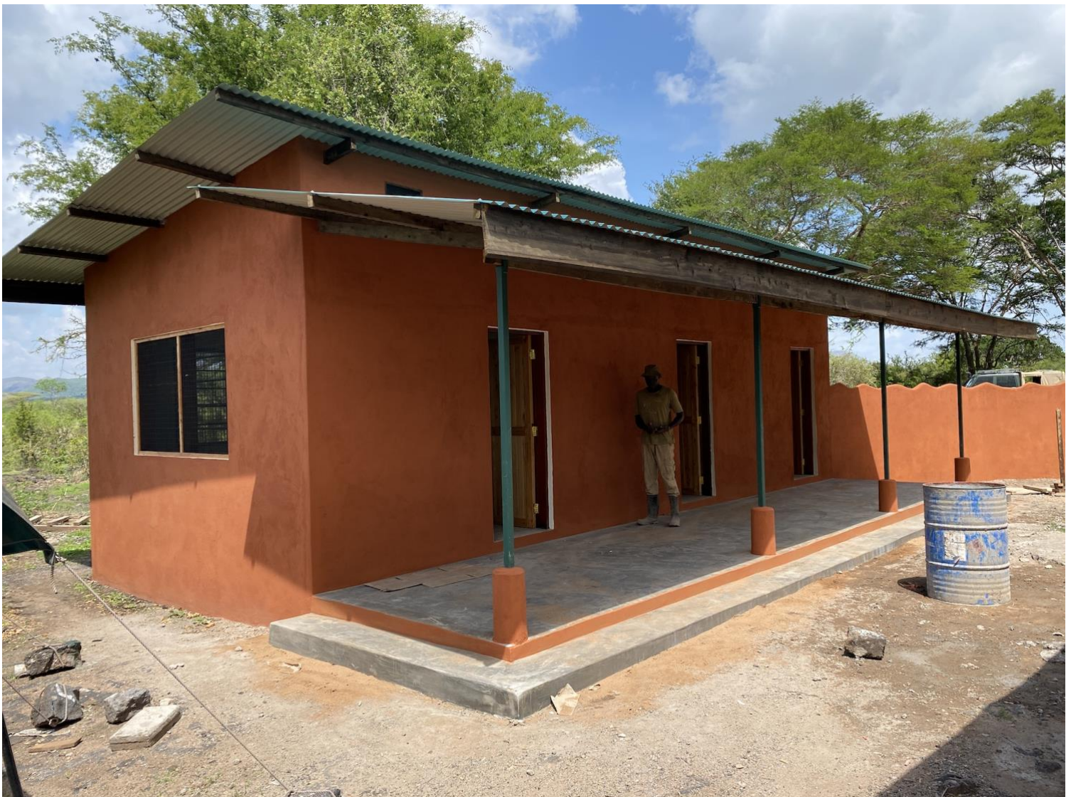
8 th December 2021: shows refurbishment of old Chyulu Gate in TWNP's IPZ as a permanent ranger outpost. Here is one of 3 ranger barracks. Included is a kitchen, ablution block, water tanks, Officers room and in early 2022 a shaded area and toilets will be completed for visitors and tourists that pass through along the main access route close by. This project, to support KWS, has been generously funded by US Fish & Wildlife Service – African Elephant Conservation Fund.
